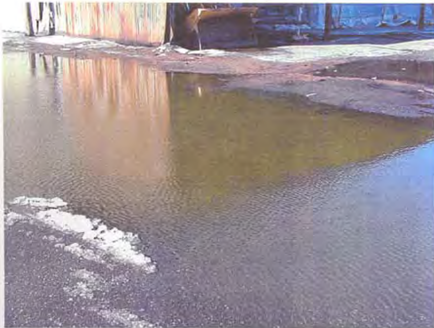
Photograph 14: Standing water as observed in the shared driveway
