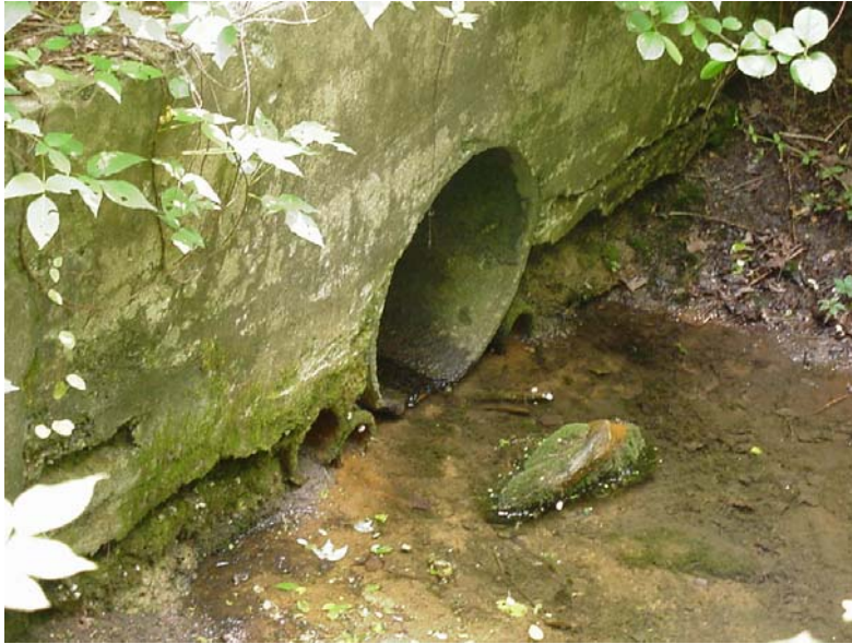
Photograph 5: Outfall pipes draining into the unnamed creek
