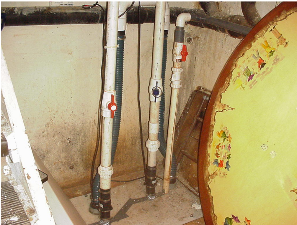
Photograph 4: Groundwater extraction and vapor head-space recovery points for the treatment system located on The City Grill property.
