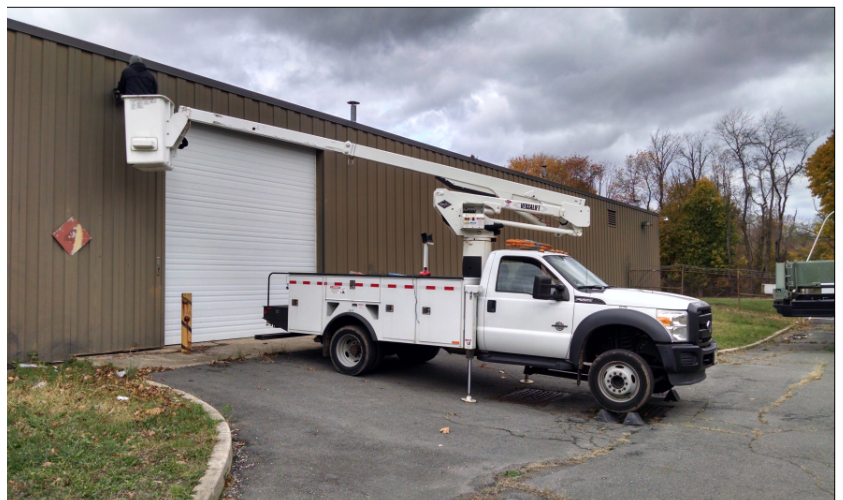
DMAVA electrician, Matthew Scudder, replaces an exterior metal halide light fixture with a new LED. The new LED will use 75% less electricity!
