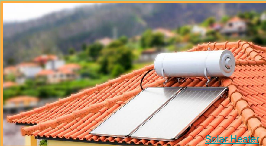
Solar water heater collector on a rooftop.
